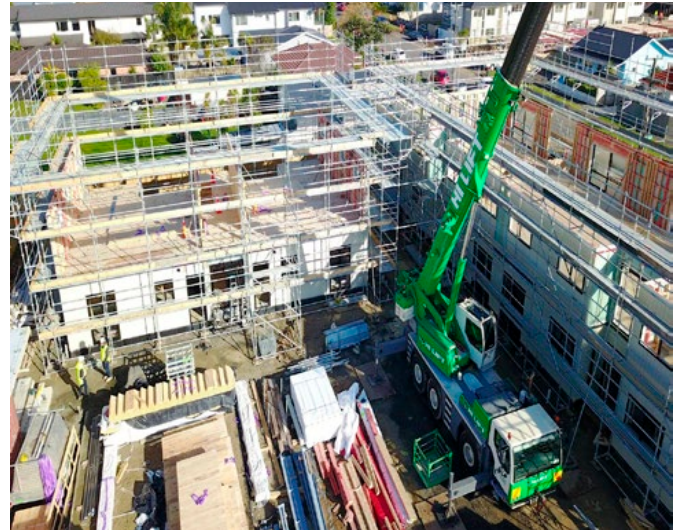
The Busby Street project utilises bathroom pods, manufactured light timber frame panels, CLT structural panels and air-stairs.
